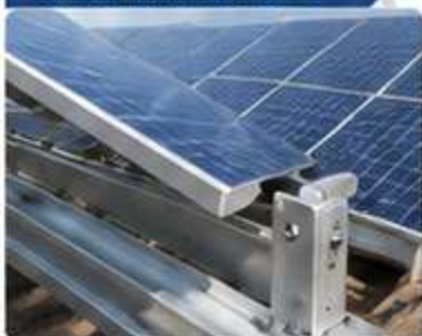
SOLAR MOUNTING STRUCTURES
