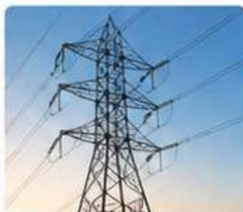
TRANSMISSION &amp; DISTRIBUTION
